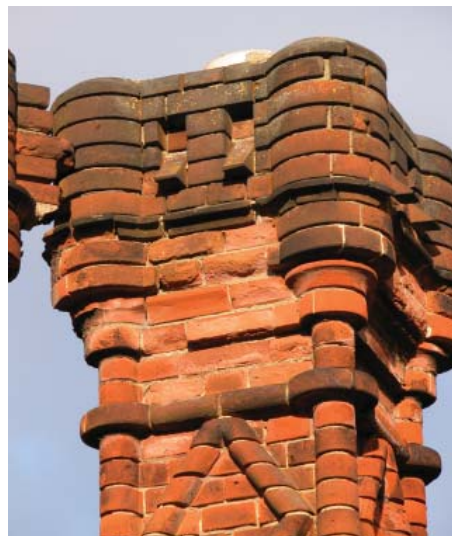
Loose and eroded brickwork before repair
